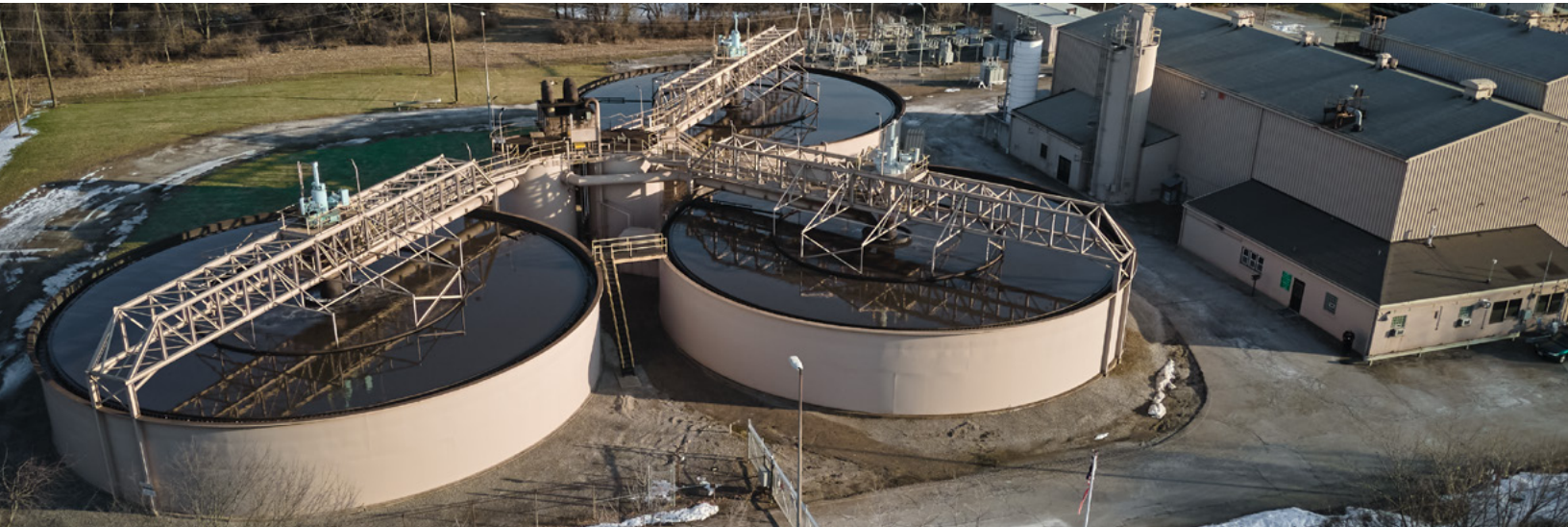
TimkenSteel's water treatment plant
